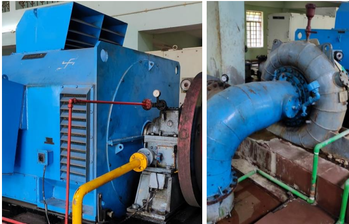
Figure-2: 3 MW Lachung Hydro Turbine inside Power House
